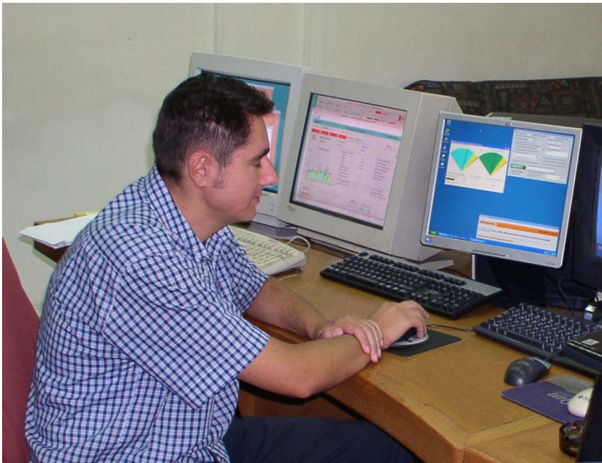
Siemens' SCADA/EMS and QuickStab® workstations side by side on the operator's console in the NOS BiH control room. The two-speedometers chart pops up automatically after each successful processing of the state estimation output.
